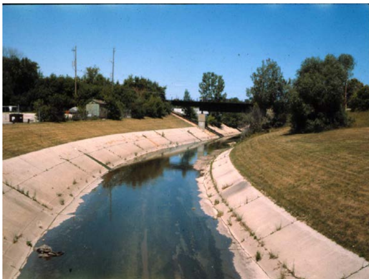
FIGURE 5-2 Concrete channel in Lincoln Creek, Milwaukee, Wisconsin. SOURCE: Roger Bannerman, Wisconsin Department of Natural Resources.
