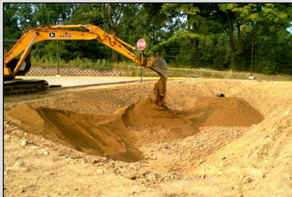
FIGURE 5-22 Placement of the mixed soil in the basin. Notice the construction equipment being kept away from the basin to avoid potential compaction of the sub-base. SOURCE: Reprinted, with permission, from VUSP. Copyright by Villanova Urban Stormwater Partnership.
