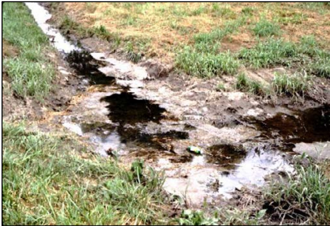
FIGURE 3-32 Failing sanitary sewer, causing upwelling of sewage through soil, and draining to gutter and then to storm drainage system. SOURCE: Robert Pitt, University of Alabama.
