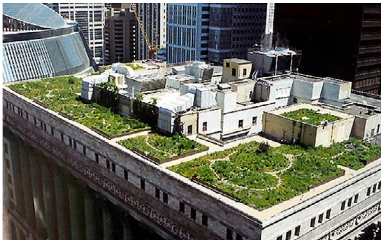
FIGURE 5-18 City Hall in the center of Chicago's downtown was retrofitted with a green roof to reduce the heat island effect, remove airborne pollutants, and attenuate stormwater flows as a demonstration of innovative stormwater management in an ultra-urban setting. SOURCE: Courtesy of the Conservation Design Forum.
