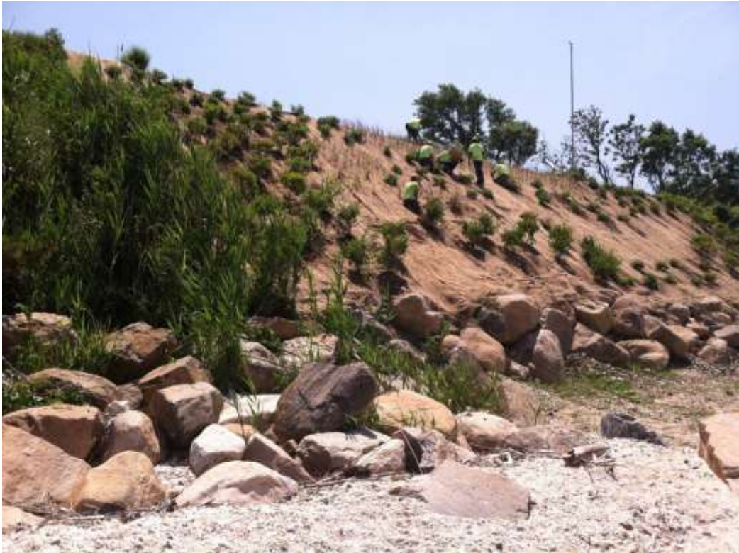
Workers at Orient Point in Suffolk County installing native vegetation and jute matting to restore an eroded coastal bluff, which is also protected by boulders at the base, or “toe” of the bluff.
