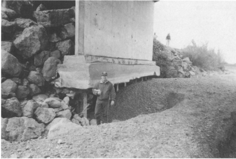
Fig. 6. Undermining of the Highway 32 bridge over Stony Creek, near Orland, California. The channel incised 5 m, necessitating repairs costing over US $1.5 million. (Photograph by the author, May 1990.)
