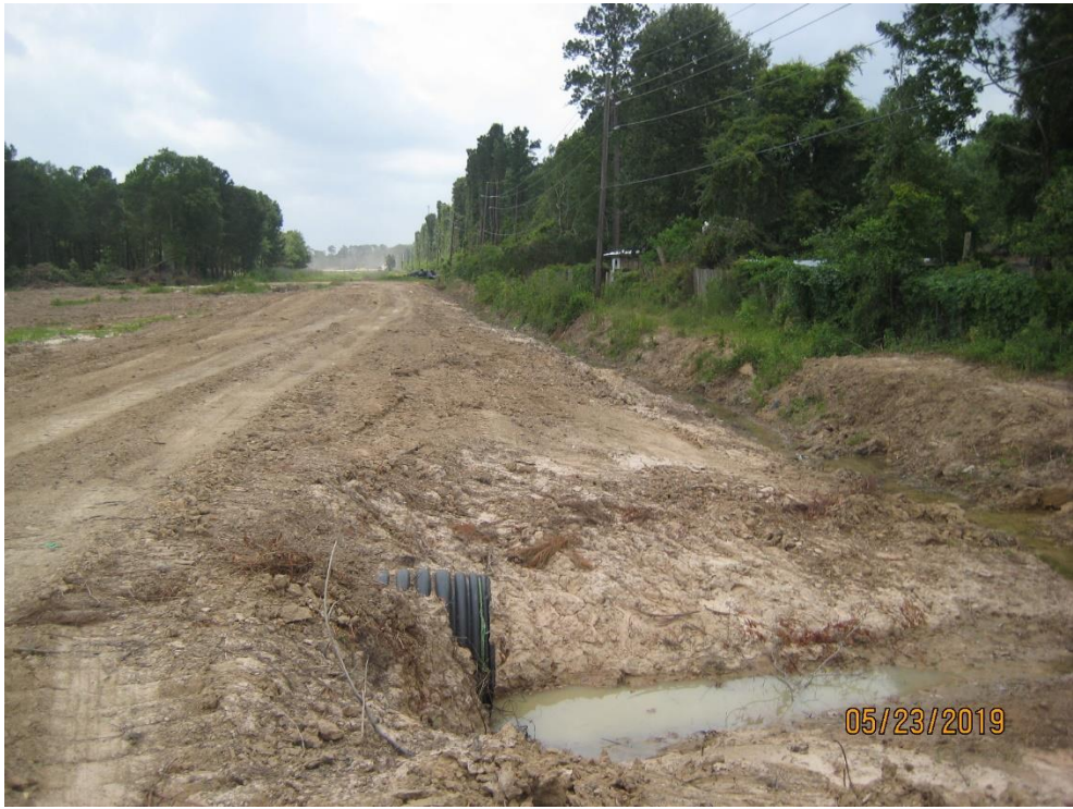
Drainage channel on west side of the northern cleared area near Webb Street; needs perimeter controls installed
