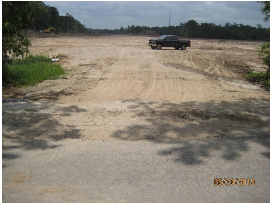
Entrance/Exit at Webb Street; needs to be stabilized with rock
