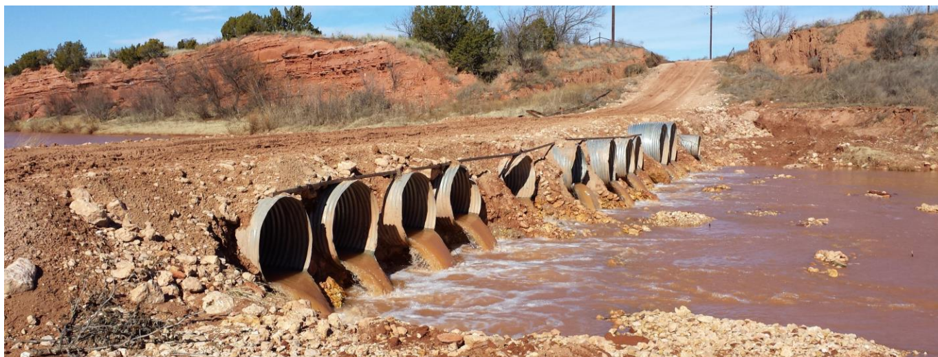
Figure 3. Unpermitted stream crossing in the southern Great Plains of Texas.
