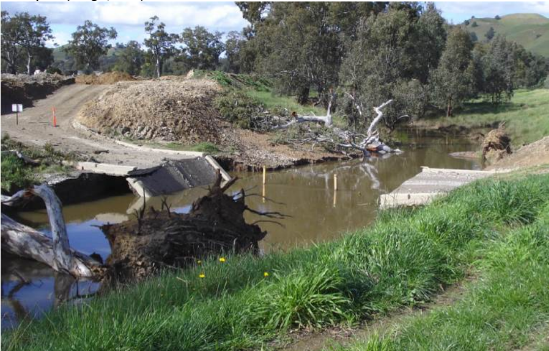
Figure 3. Road crossing in Figure 2 destroyed by bed incision which has also toppled riparian trees (Craigie, 2012)
